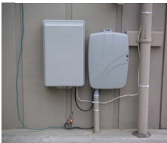
A typical installation at a member's premise which includes a battery supply (left) and an optical network terminal (right) which provides services into your home.
