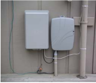
A typical installation at a member's premise which includes a battery supply (left) and an optical network terminal (right) which provides services into your home.
