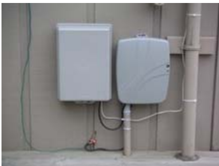
A Typical Installation Battery Power Supply (left) and Optical Network Terminal (ONT) (right)
